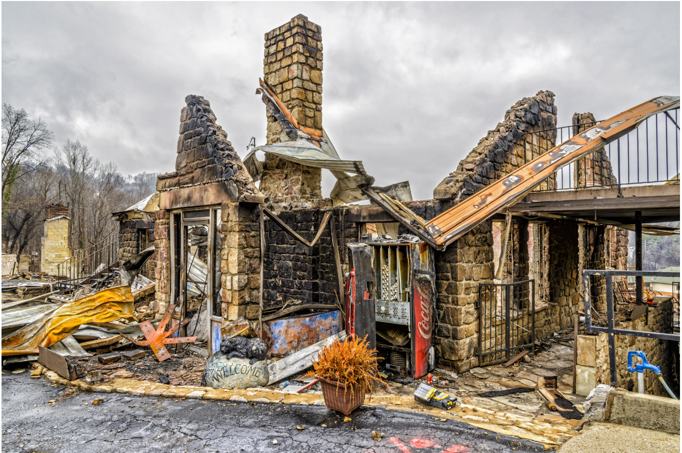
Only the shell of a motel office remains after being destroyed by a forest fire in Gatlinburg and the Smoky Mountains in late 2016.
